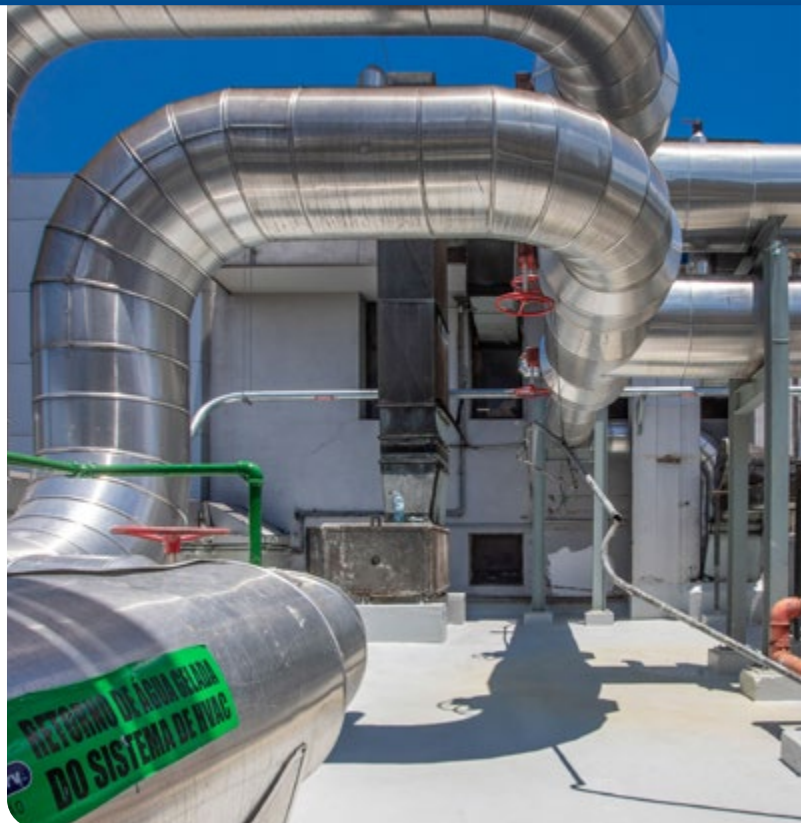
↑ The new Morumbi Chilled Water Center provides the cooling of operating theatres and inpatient areas, with precise, safe and economical thermal control
