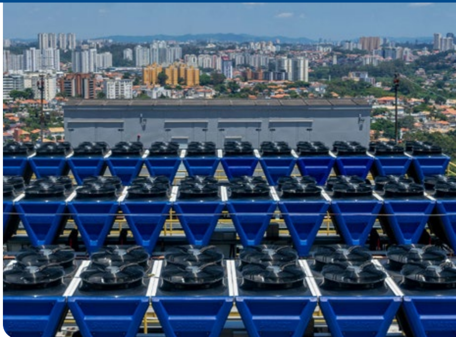
↑Morumbi Chilled Water Center
