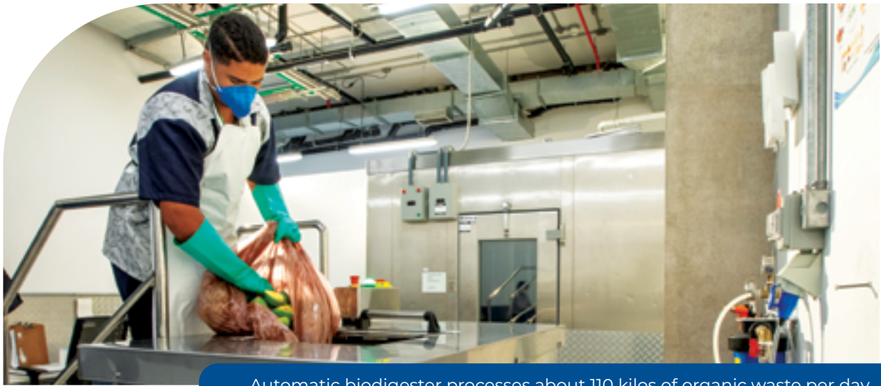
Automatic biodigester processes about 110 kilos of organic waste per day
