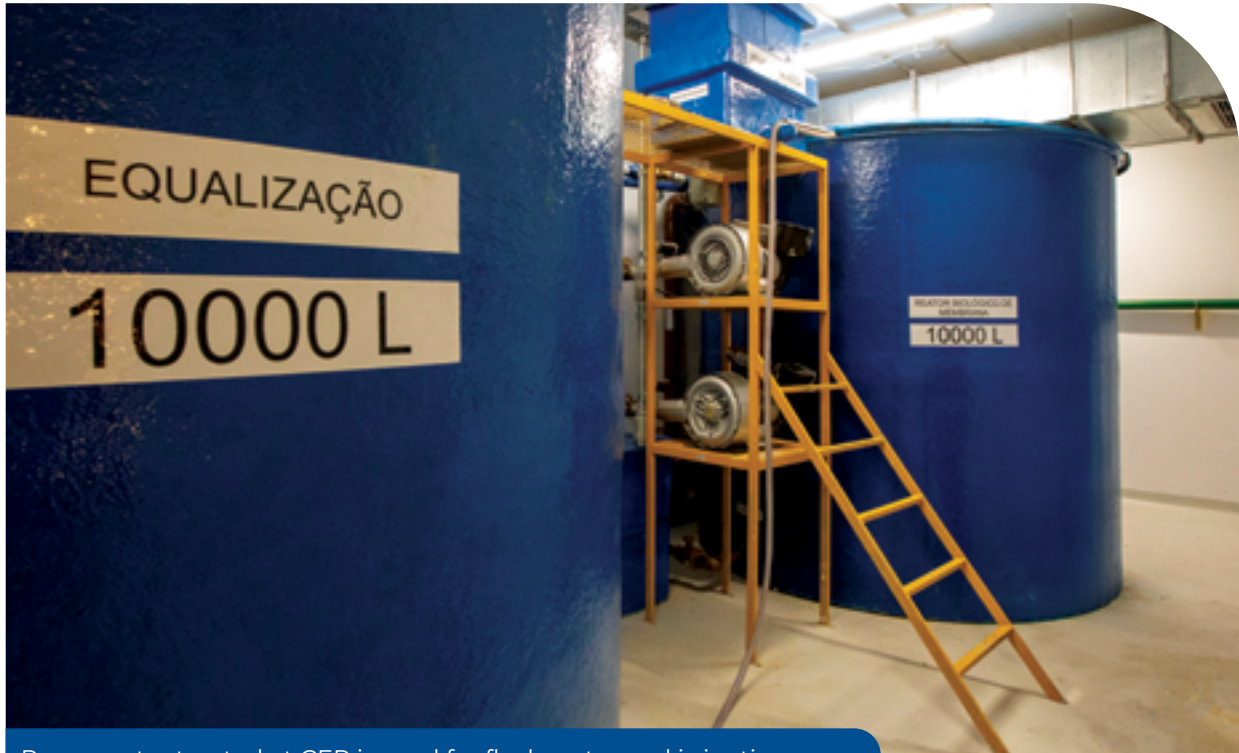
Reuse water treated at CEP is used for flush water and irrigation
