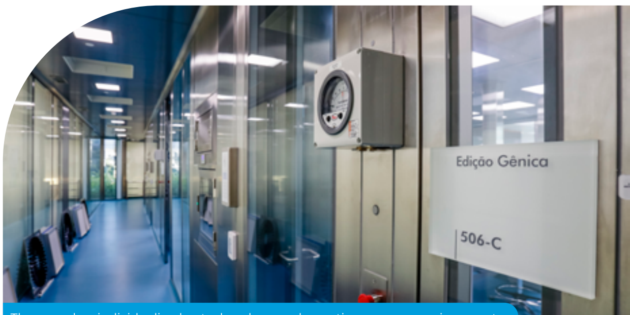
The room has individualized antechambers and negative pressure environments
