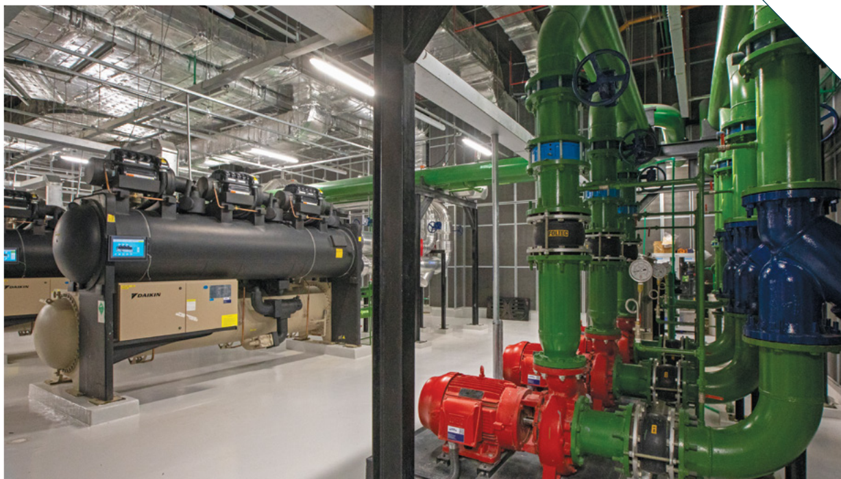
Chilled water plant for cooling the environments of the Teaching and Research Center
